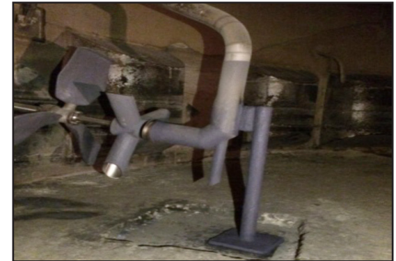
Design was modified to include additional support for the mixer and lance
